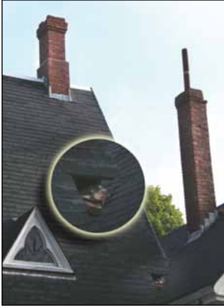
One of the four Chimnies that desperately need a rebuild at the Ellis House... note the fallen bricks int he eaves!
